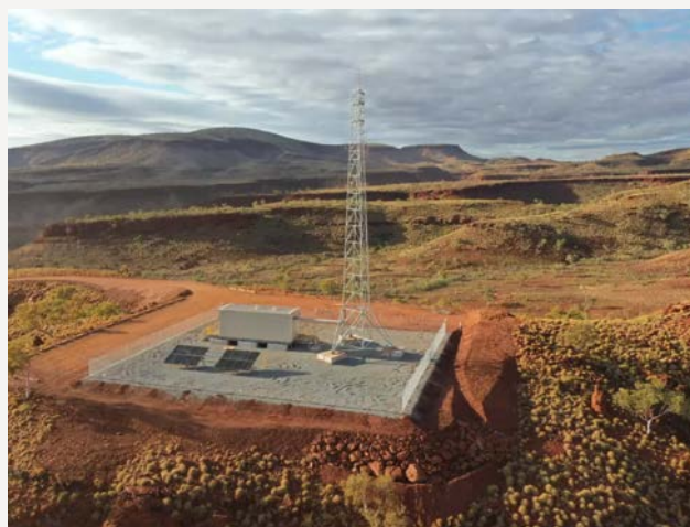
One of Radlink's telecommunications towers
